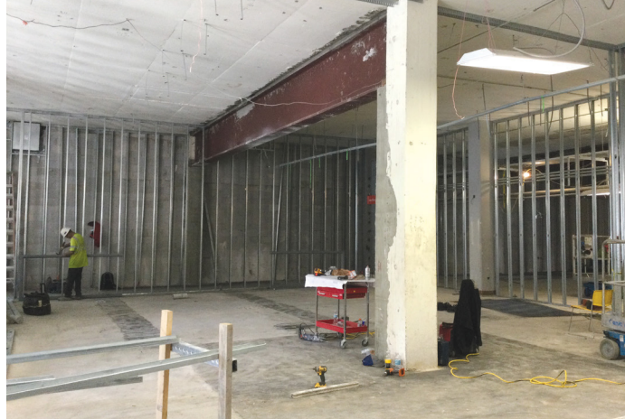
Two cast-in-place concrete columns were removed and replaced with new steel transfer beams as part of the Centrex Building reconstruction.
