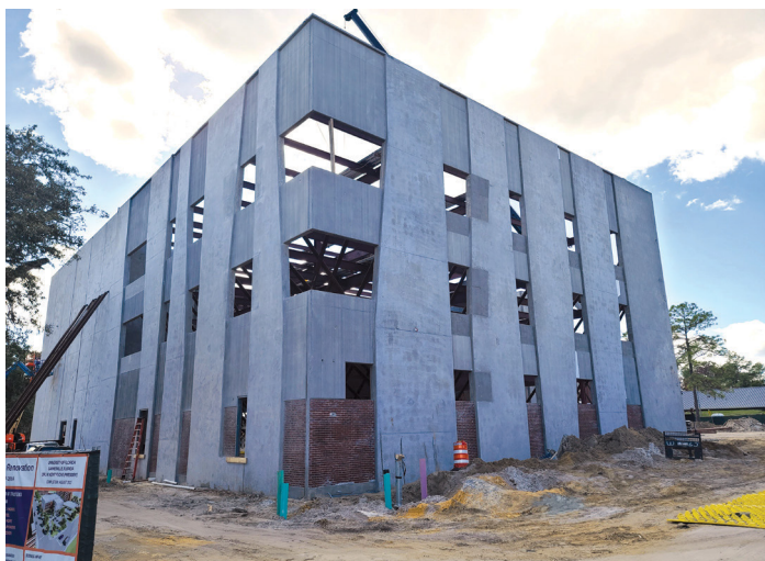
A unique component of the tilt wall design is the blend of architectural and structural design
