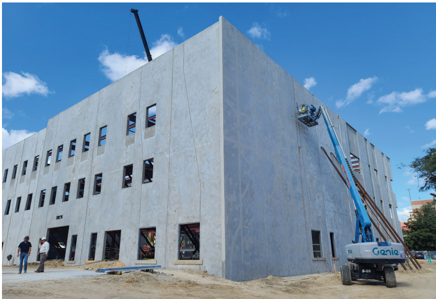
The University of Florida Public Safety Building is located in the middle of campus and constructed using tilt-up concrete wall panels for the exterior structure.
